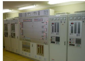
Electrical Services at RAAF Edinburgh
